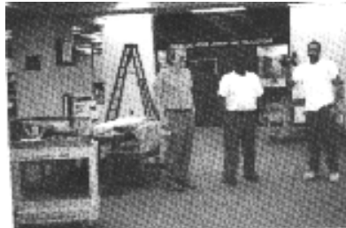
The CSU carpenter crew working on the construction of the Special Collections wall.
