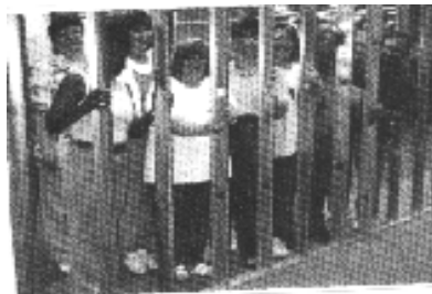
Some members of the Library staff checking the progress of wall's construction.
